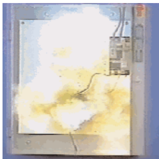
Photo 2: Same as Photo 1, but during the test with MCP as the motor branch circuit protection. The heater elements vaporized and the contacts were severely welded. Extensive starter repair or total starter replacement would be required. This level of damage is permissible by UL508 or UL508E/IEC60947-4-1 Type 1 protection.
